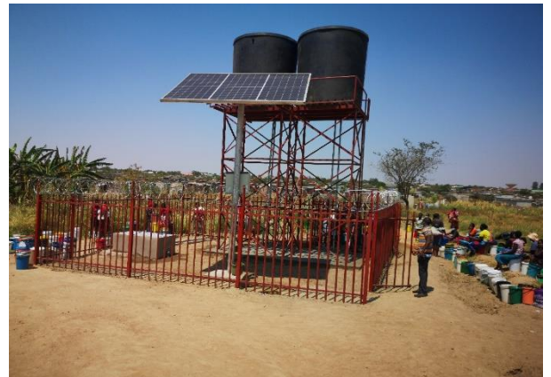
Picture showing the whole Piped Water Scheme Structure at Hopley Borehole 1 as beneficiaries access water.
